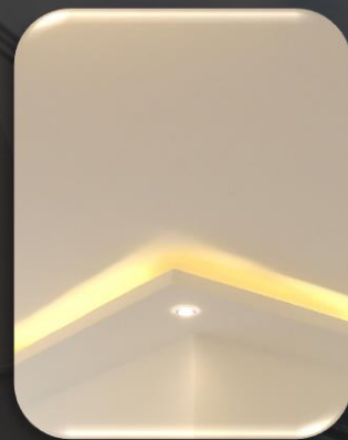
Indirect LED Lighting
